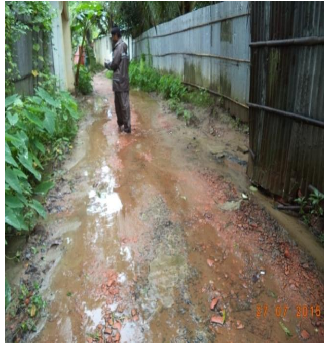
Existing damaged narrow road
