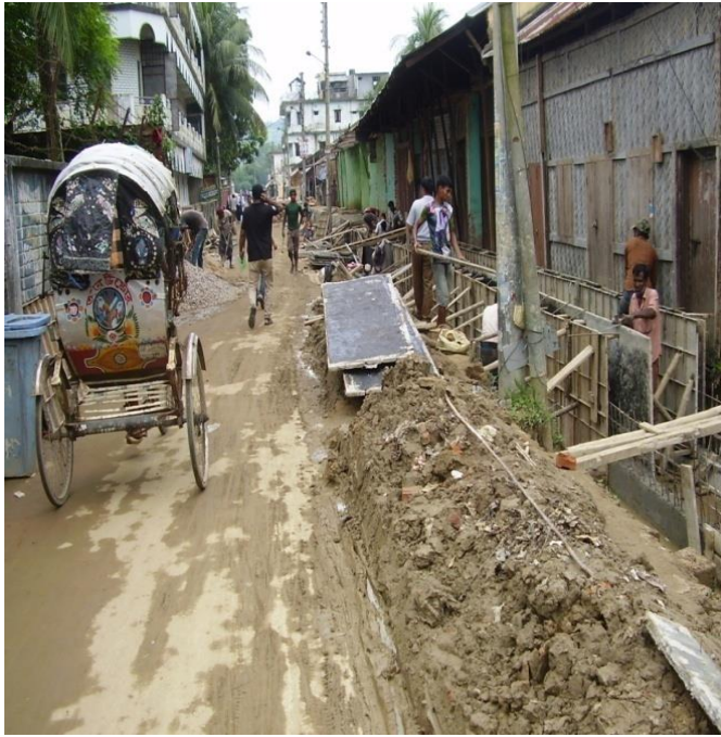
Existing damaged road
