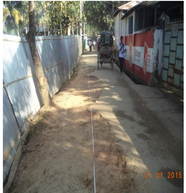
Existing damaged narrow road
